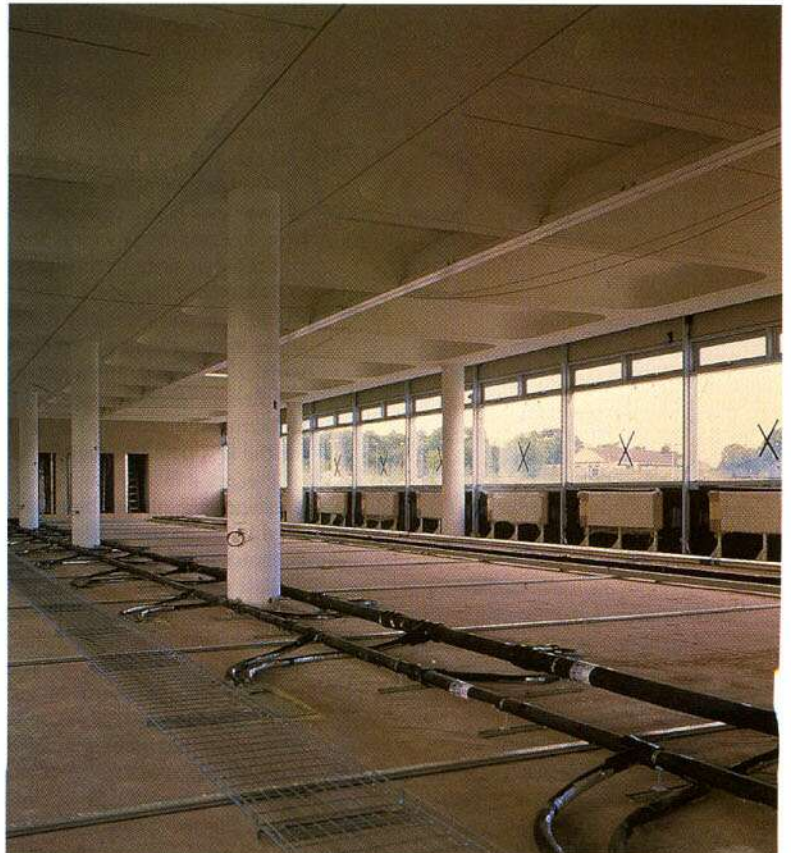
The pipework and coffer are already in place, waiting for the rest of the fit-out.
